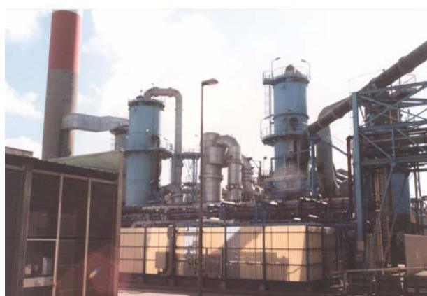
Fig. 2 TIOXIDE sulphuric acid recovery plant
