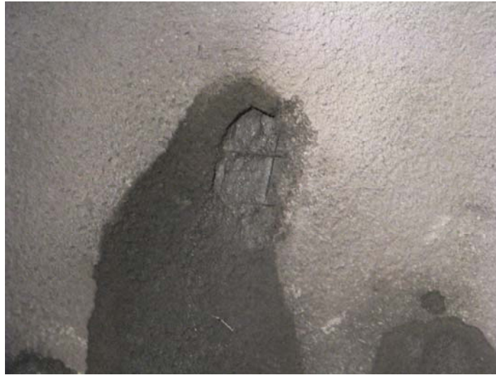
Fig. 12: Typical damage to unmodified sprayed concrete due to formation water pressure
