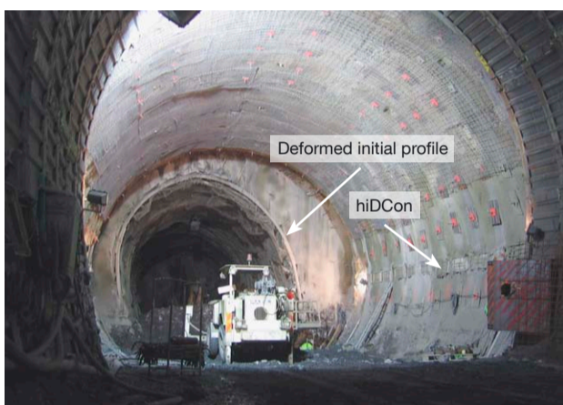
Saint Martin la Porte access tunnel, change from stiff to yielding support (source: Razel/Bilfinger Berger/Pizzarotti)
