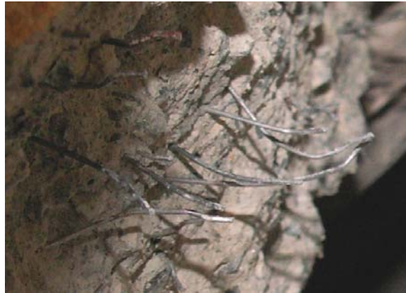
Figure 12: Steel fibres showed no signs of tensile yield.
