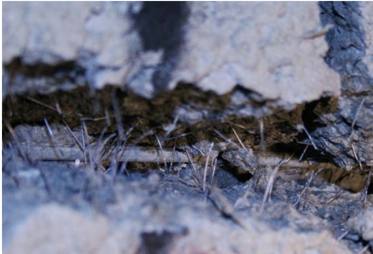
Figure 14: Mesh reinforcing within the cracked shotcrete sample.
