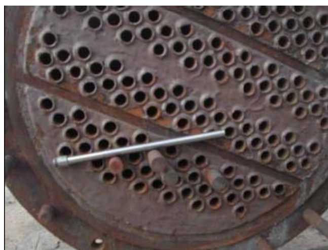
Fig.4: Clean H 2 S Cooler by CQM's ATCS
