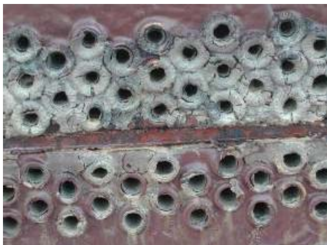
Fig 2: Clogged H 2 S Cooler: mud and scale
