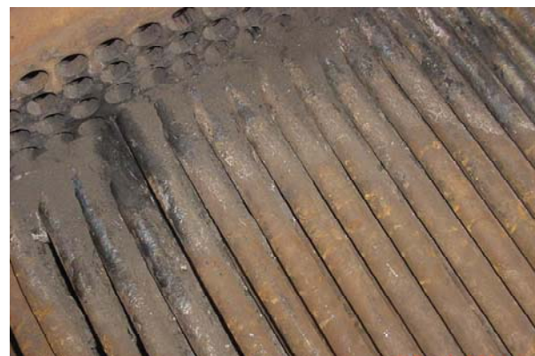
Fig. 1-a) Fouling Accumulation on the Tubes
