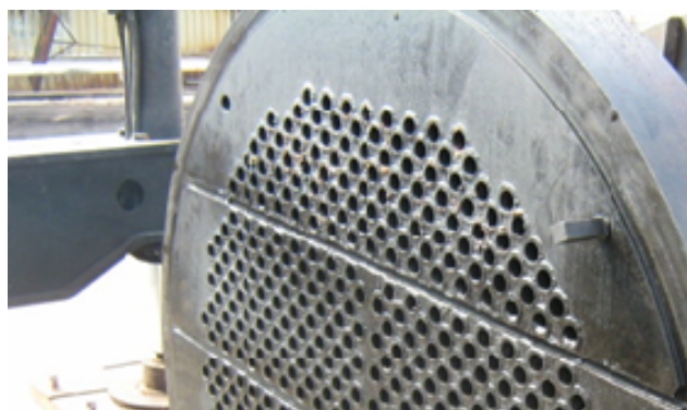
Figure 6. Visual Observation for Heat Exchanger B
