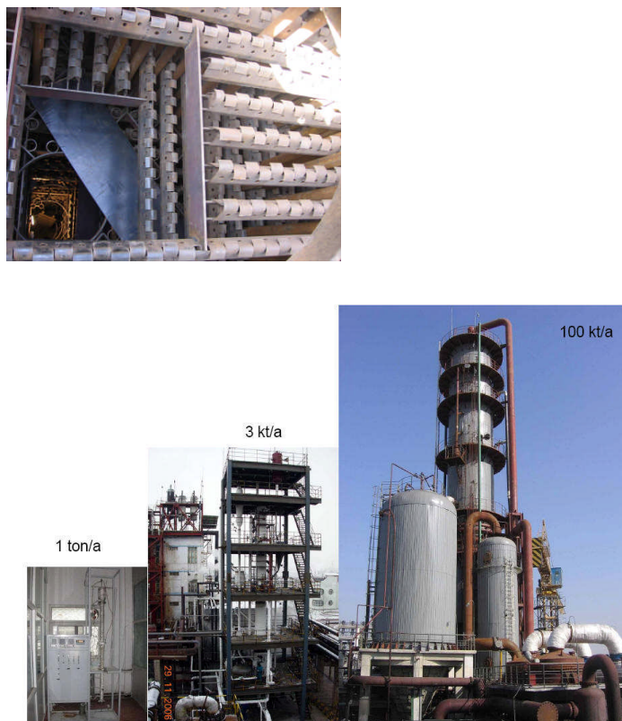
Fig. 8. Top: Internal structured fluidized bed reaction; Bottom: Multistage fluidized bed reactor for VCM production scale-up process: Left: small hot model test unit; Middle: 3 kT/a pilot plant; Right: 100kT/a multistage fluidized bed CVM unit
