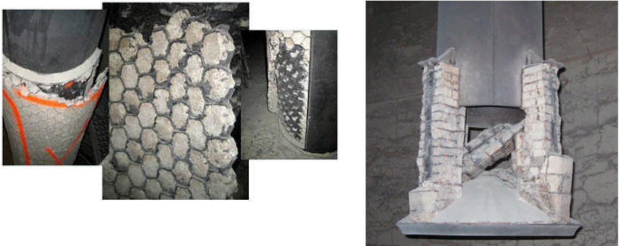
Figure 10. (a) Failed refractory, in sheets, due to Hex Mesh corrosion [6]; (b): fallen refract sheets caught above the primary cyclone termination device
