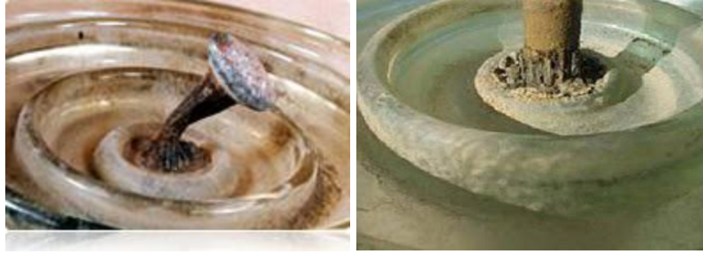
Fig 1.6. Corroded pins in suspension-type porcelain and glass insulators [16].
