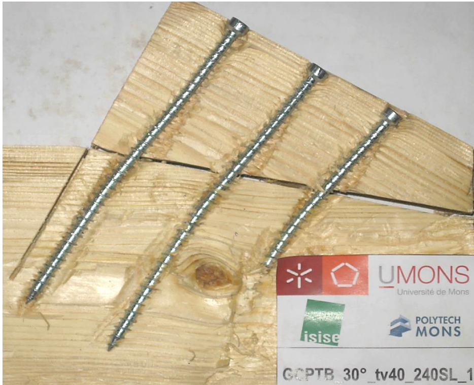
Fig. 11 Plastic hinges of FTS implemented in the rafter at the bottom-notch surface.
