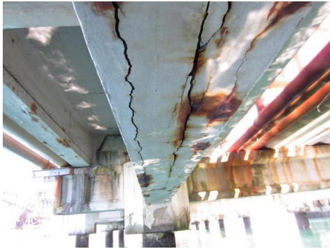
Figure 1. Longitudinal cracks in the bottom flange of the beam
