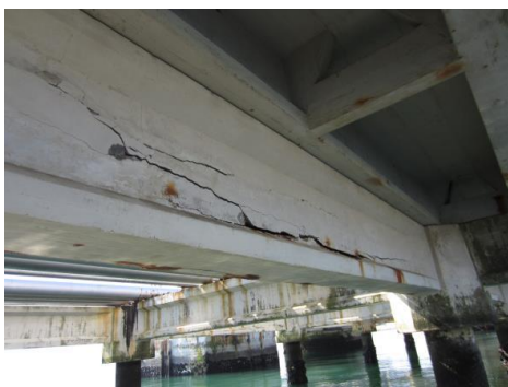
Figure 2. Longitudinal cracks in the core of the beam associated with the pre-stress cables
