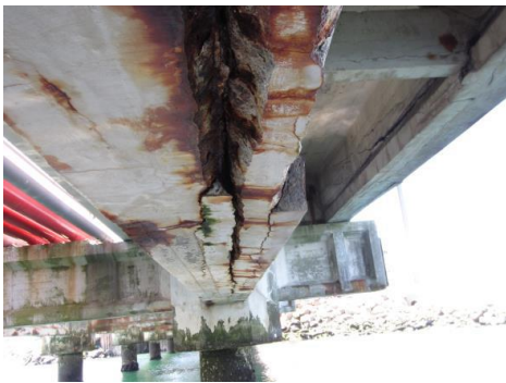
Figure 3. Loss of section associated with the corrosion of the reinforcement
