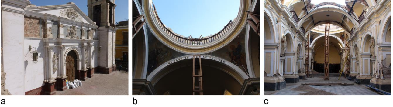
Fig. 1 Ica Cathedral damage after the earthquakes in 2007 and 2009: a front façade, b main dome at transept, c barrel vaults with lunettes and pillars
