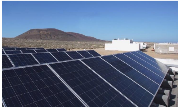
Figure 98: Example of PV modules installed in the island.
