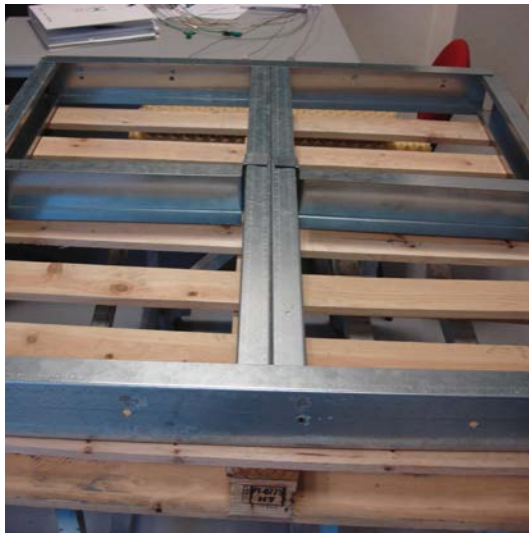
(a) Structure in Specimen 6.
