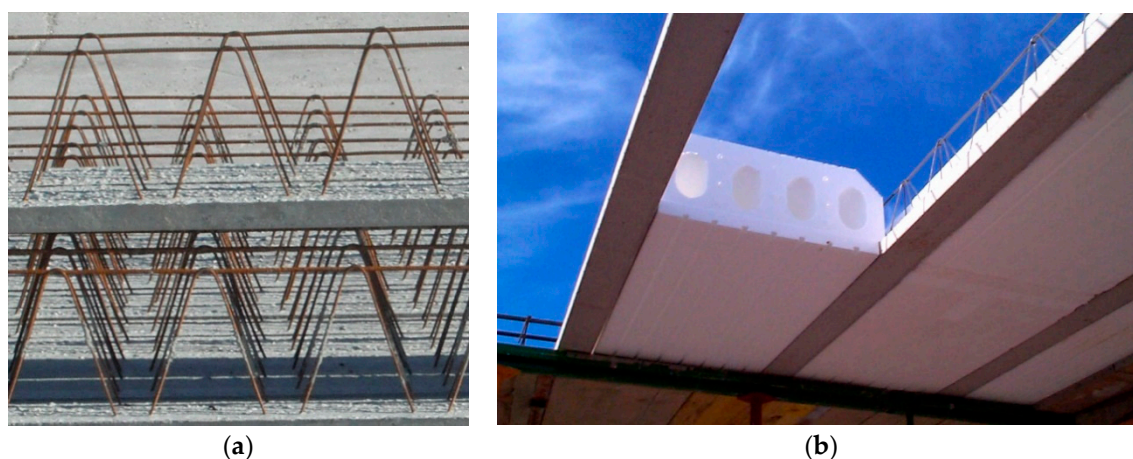
Figure 1. Reinforced RC joists (without pre-stressing) are commonly used in northern Spain areas: (a) lateral view of typical RC joists; and (b) general view of the one-way ribbed slabs, source: Iberacerros Forjados Riojanos, [4].
