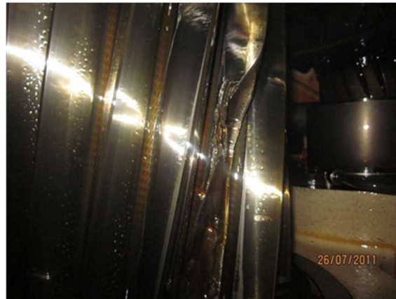
Figure 13. Photograph of gear 2 at intermediate shaft with a broken teeth found out during inspection.
