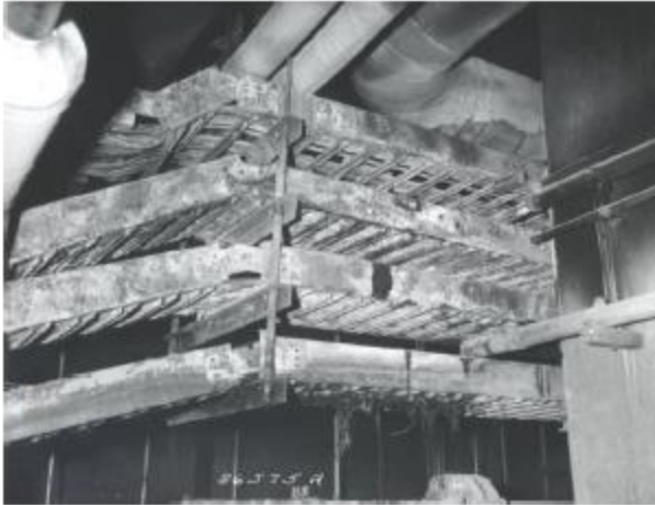
Figure 4.1 Brown Ferry cable trays after the fire, showing damaged cables [24]
