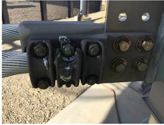
Figure 1.8: Failed substation connector.
