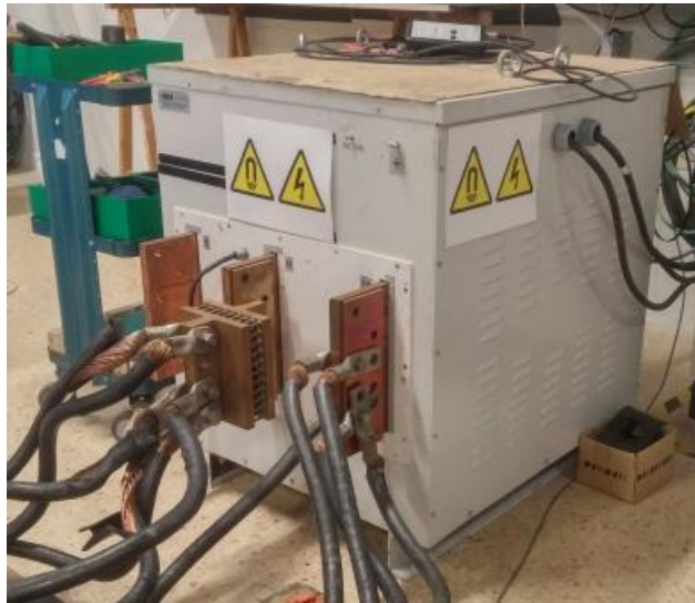
Figure 1.4: High-current transformer used in Temperature rise tests and reduced-scale short-circuits
