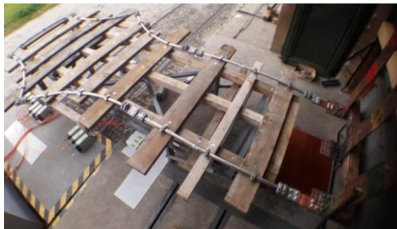
Figure 2.14: Short-circuit tests. Test loop composed of HTLS conductors and S285TLS T-type connectors.
