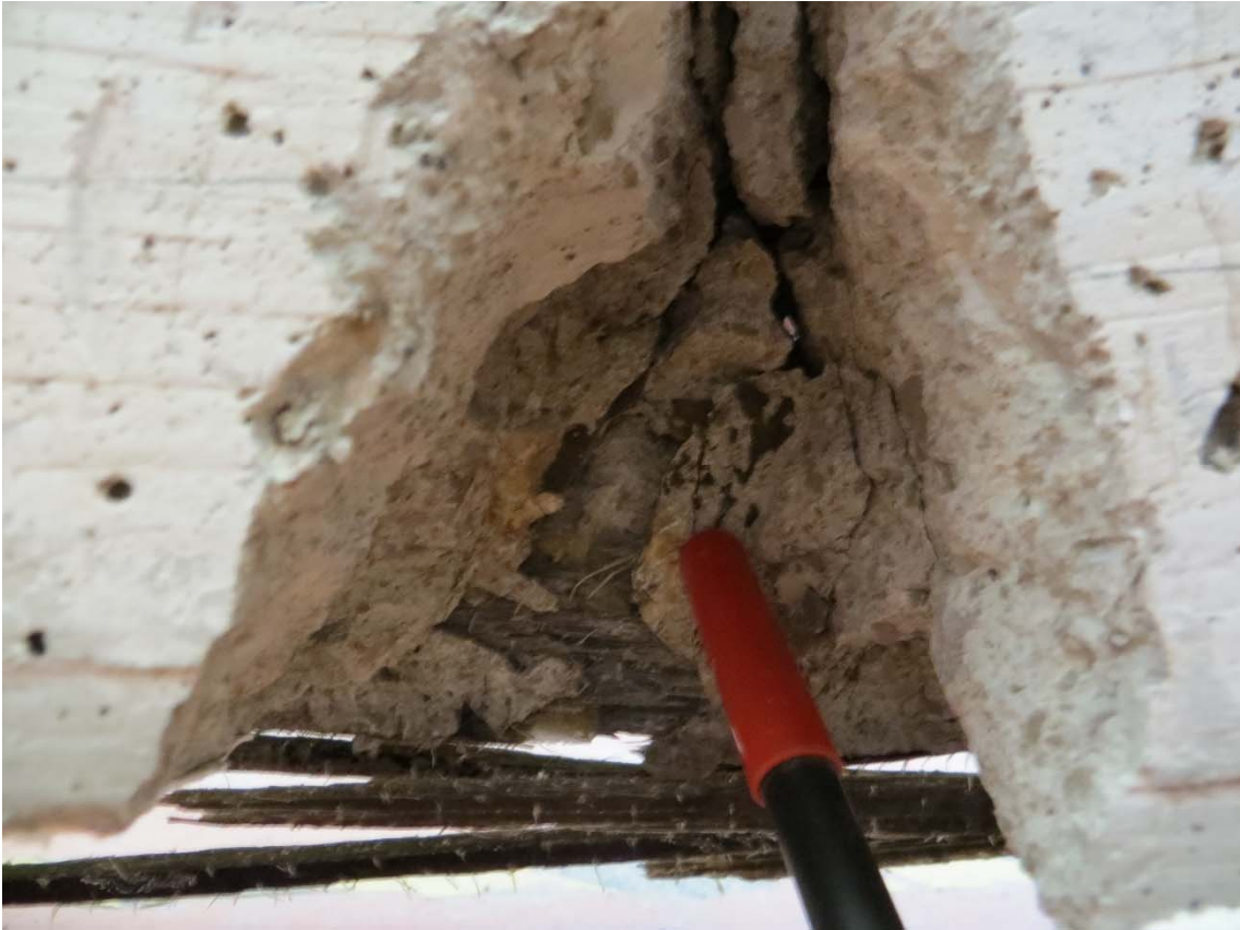
Figure 19. Failure of the laminate FRP-control beam
