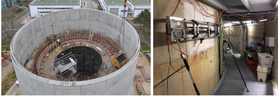
(a) The two containments during construction (b) Internal corridor with the view of the internal and external walls
