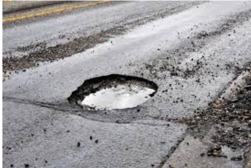
Figure 1.1: A pothole in a road.
