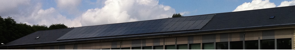
Image 4: Solar panels on the school roof
