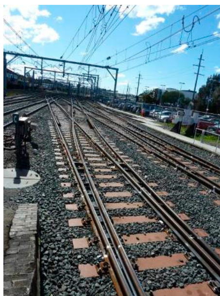
Figure 4. General condition of the double slips.
