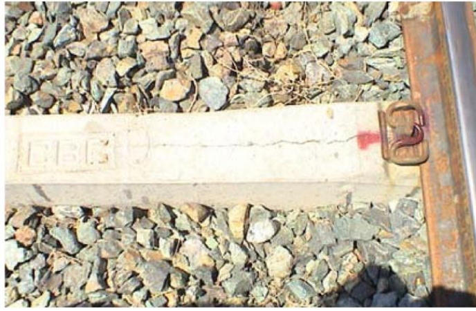
760 761 Figure 6. Longitudinal cracks in concrete sleepers (Rezaie, Bayat, and Farnam 2016) 762 763
