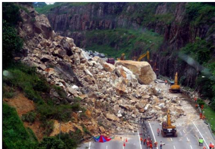
Figure 15. The Bukit Lanjan rockfall along the New Klang Valley Expressway in November 2003 resulted in a six-month closure of that particular stretch (Courtesy: Malaysia Department of Public Works).
