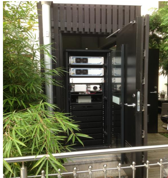
Fig. 3 Smart Energy Storage System Installed in Western Harbour
