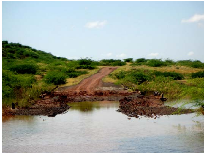
The 30km length narrow road connecting the village to the Taluka broken and drowned during monsoon (first author)
