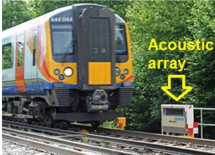
Figure 4: A RailBAM trackside acoustic array detector installed on the British rail network near London (the photograph is courtesy of SIEMENS).
