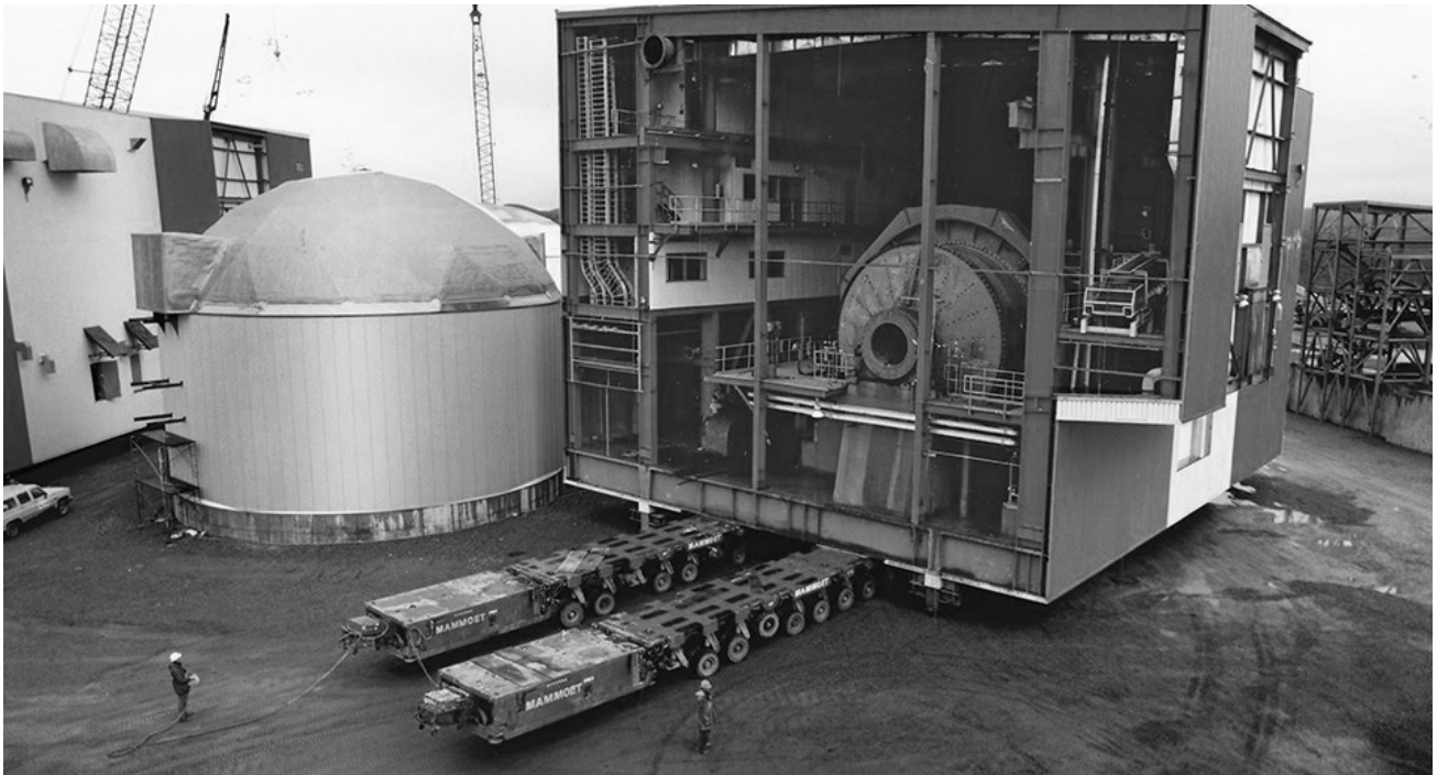
Figure 1: Heavy equipment being transported on a platform composed of Self-Propelled Modular Transporters (SPMTs), Courtesy of and ® of Mammoet (2015b).
