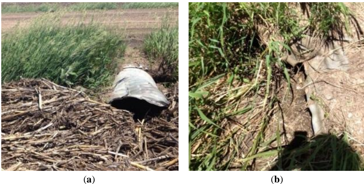
Figure 6. Culverts silted by (a) corn stalks and (b) sedimentation.
