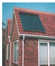
Solar hot water
