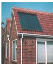
Solar hot water
