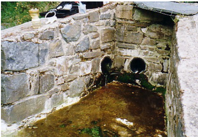
Figure 2.9. Outlet pipes at Bwlch.
