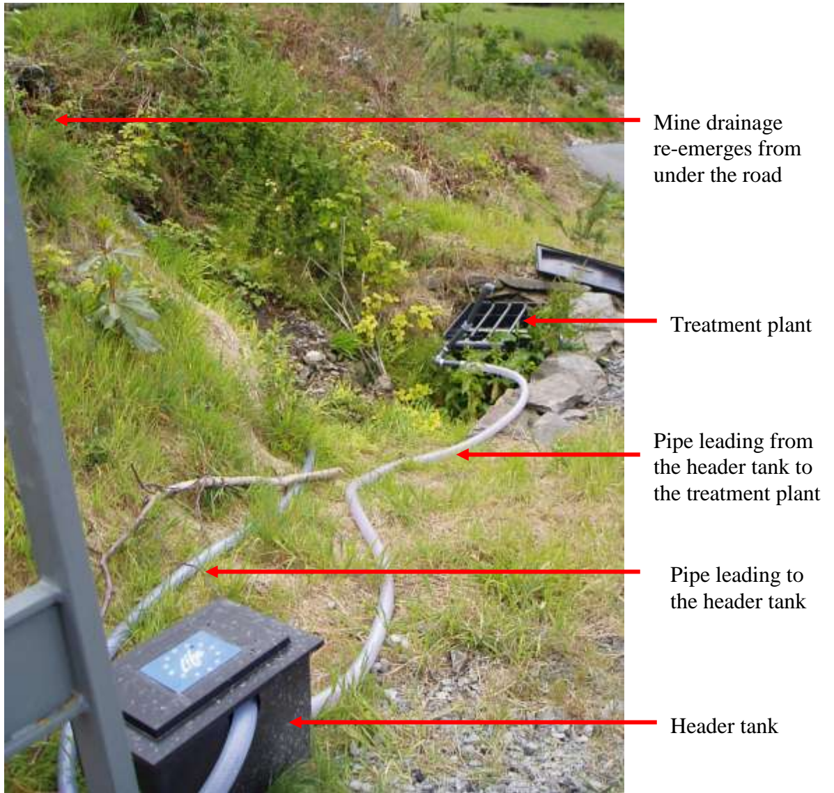
Figure 7.25. Alltycrib treatment plant
