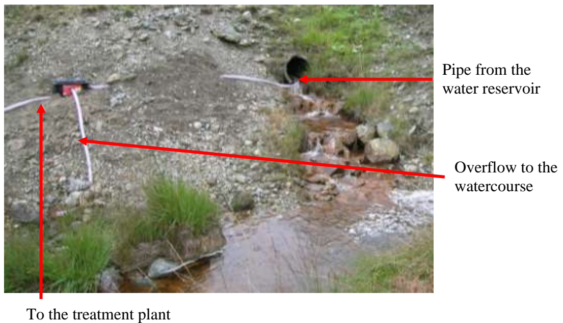
Figure 7.14. Header tank for the Esgair Hir treatment plant.
