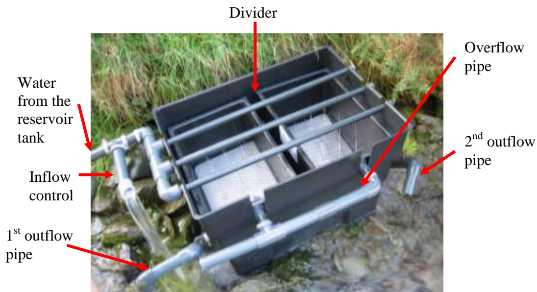
Figure 7.28. Dual treatment plant at Bwlch.
