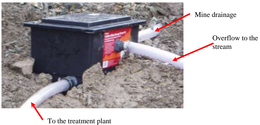
Figure 7.4. Header tank at Esgair Hir.
