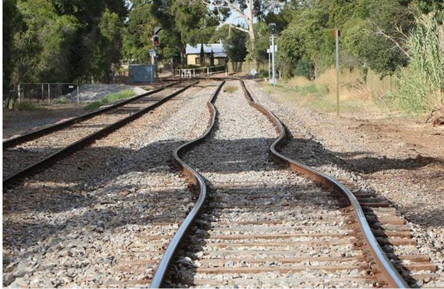
Figure 1-3 Buckling of CWRs [58]
