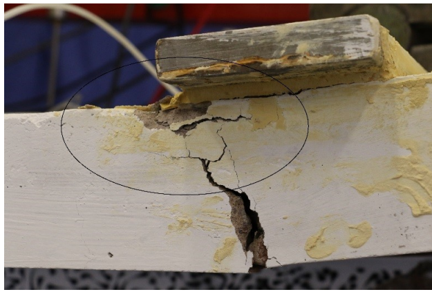
(a) Concrete crushing in T2-2
