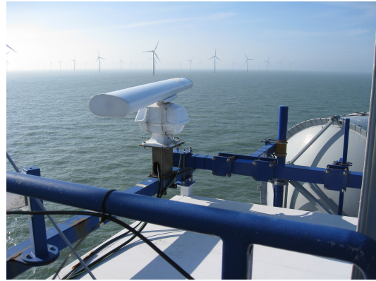
(b) Another LAWR is installed at the Horns Rev 1 wind farm for the needs of a separate experiment.
