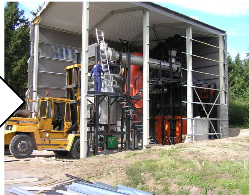
Pilot plant at Weiss A/S 1:10
