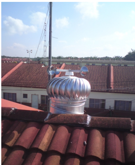
Figure 4: Prototype development and Installation [6]
