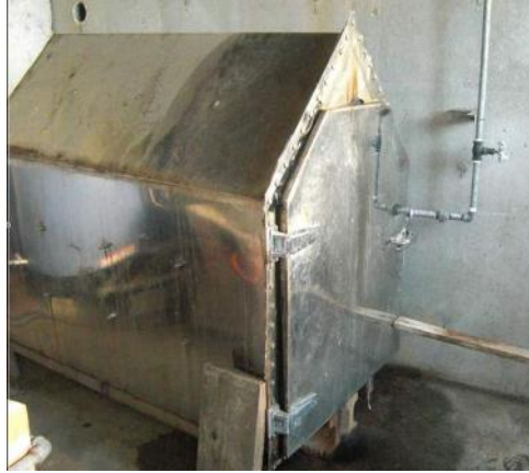
Figure 3.10: Pressure steamer inside a small shed. The steamer is made of stainless steel, with a locking door-like lid at the front
