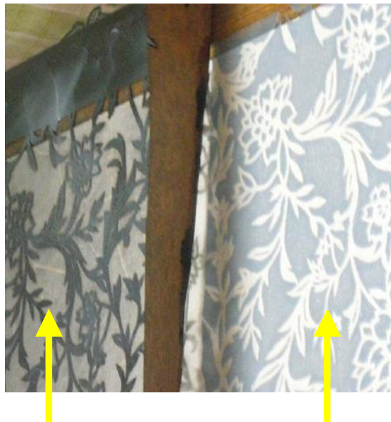
No gap between the two different surfaces
