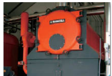
Figura 62: Caldera de biomassa per District Heating (850 kW). Font: IDAE
