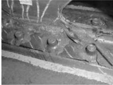
Figure 4. Assembly fastener pull-through due to hydraulic ram effects. Reproduced from BAE Systems © 2009.
