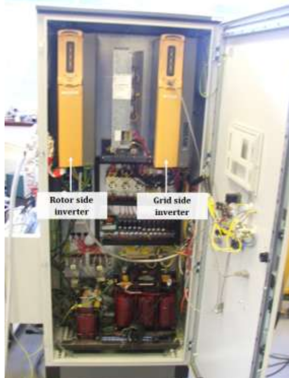
Fig. 3.4: Photographs of back-to-back converter cabinet
