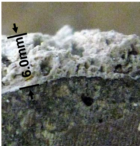
Photo 4 Surface of mortar with river sand
