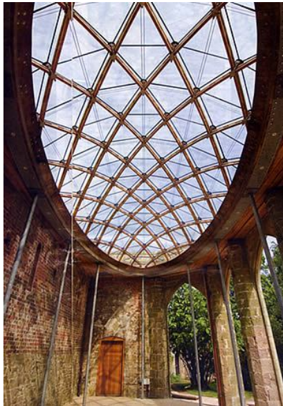
Figure A.8: Chiddingstone orangery: arch. Peter Hulbert, Engineer: Buro Happold ( photo: Carpenter Oak & Woodland Limited )
