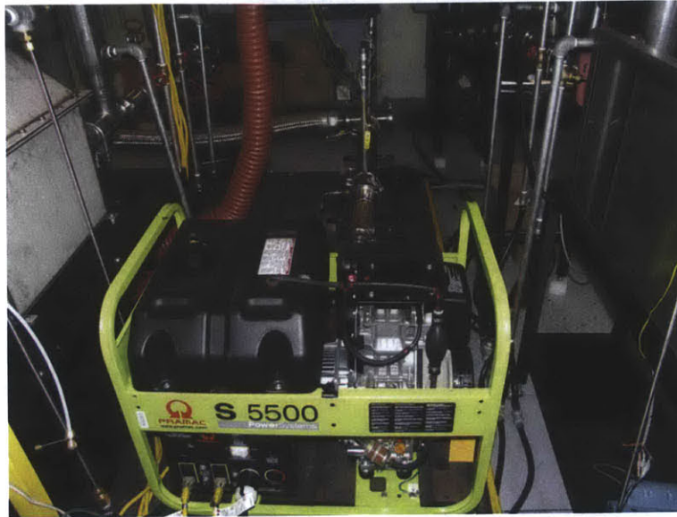
Figure 30: Pramac S5500 Yanmar L100V generator
