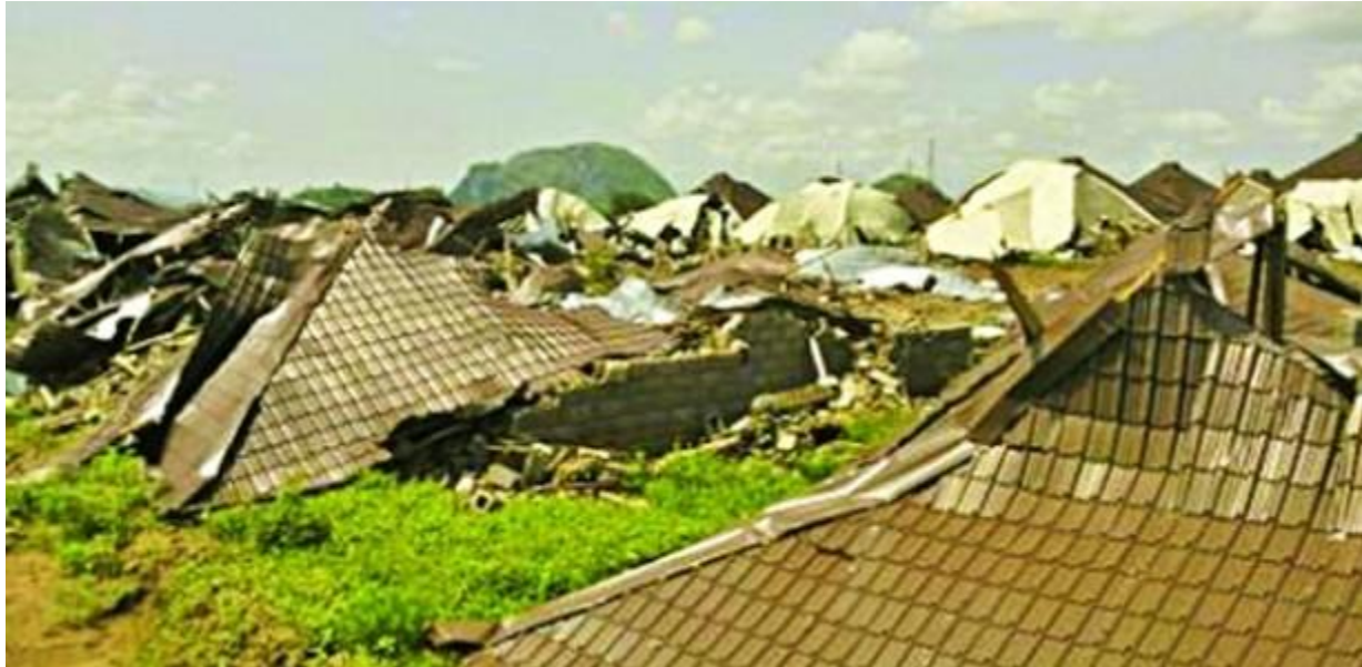
PLATE 1: A view of part of the demolished 500 housing unit in Abuja. (The SUN, 2012) [8].
