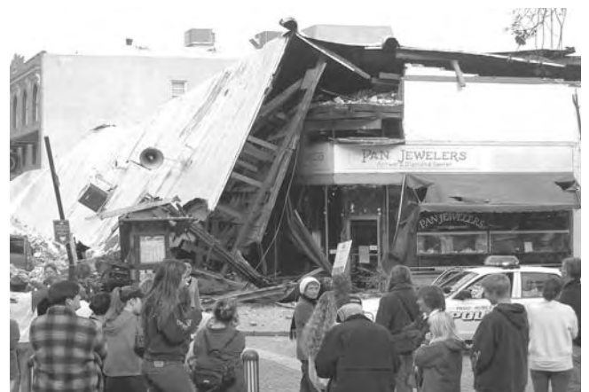
The Acorn Building in Paso Robles, after the San Simeon earthquake, 2003. (Photo: D. Stanfield)
