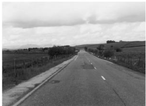
Fig. 1 : Road settlement at Cerrigydrudion, North Wales. [5]
