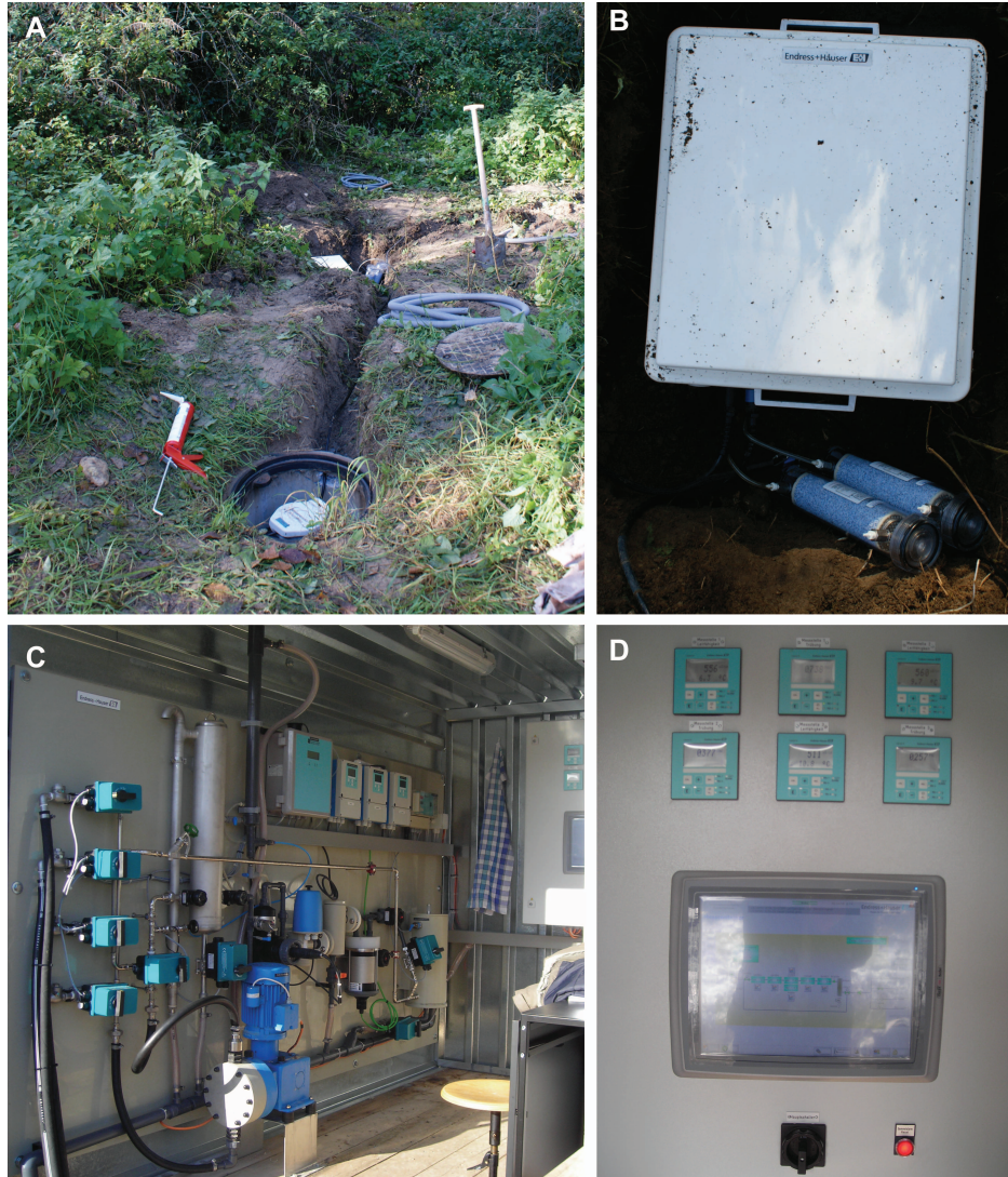
Figure 8: Two telemetry stations. Panels A and B show the stand-alone installation for data transmission from observation wells W1 and W3. Panels C and D show the container and the touch-screen of the control system (same as remote access view).
