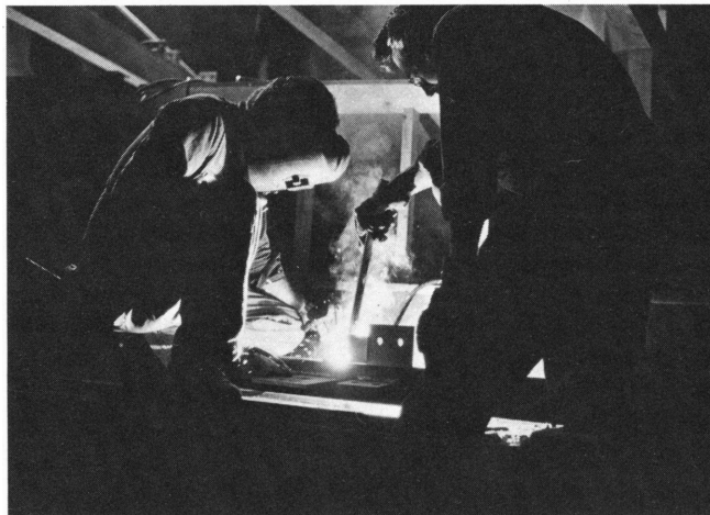
Museum workers construct a booth in the Auditorium to house a 10-foot by 12-foot IMAX projector. With the addition of a four-story retractable screen, this projector and a six-directional sound system, the Auditorium will be equipped to show the spectacular film, "To Fly." This 27-minute film depicts the history of aviation in America through scenes which show the inventiveness of the American people and the country's grandeur. Viewers experience the sensation of flight. As with the IMAX project, much of the Museum's design work and construction is done in-house by the Department of Plant Operations, Maintenance and Construction.
